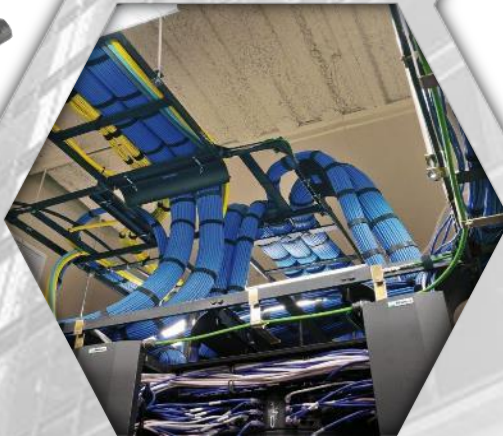
Cabling and Cable Management
